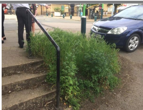
At point C where bollards would be installed to protect the slope from parking
