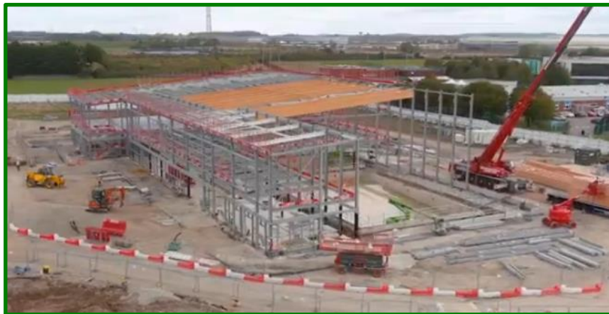
Installation of the glulam beams at the Houghton Regis Community Wellbeing Hub
